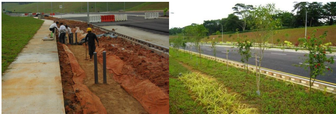
Figure 2. The Sengkang West Way road construction project to demonstrate the implementation of road side bioretention systems.
