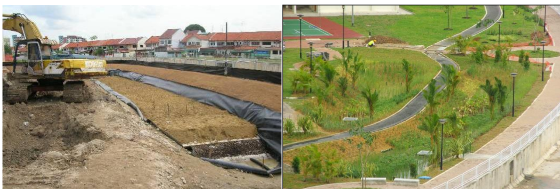
Figure 3. A 240 m 2 bioretention rain garden has been proposed and designed to capture and treat stormwater runoff from its 0.6ha contributing residential areas in Balam Estate.
